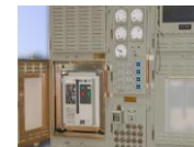
Power Conversion, & Distribution
